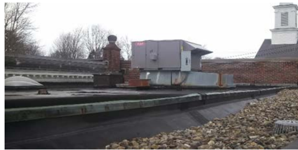
Roof air-handlers at the end of their life span.
