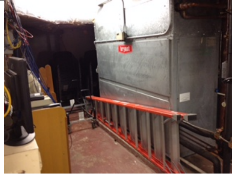
HVAC unit in boiler room at the end of its expected life cycle.
